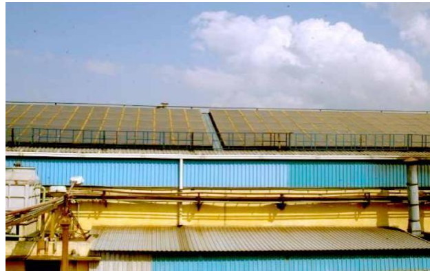
297 m 2 Solar air heating system at TI cycles in Ambattur Chennai
